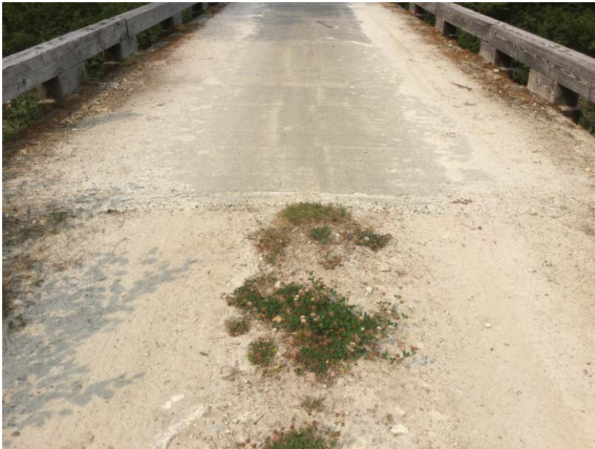
Minor damage to right bank ballast wall on wheel path
